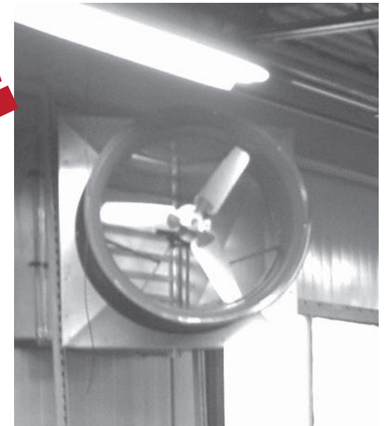
High Velocity Fresh Air Intake Fans
